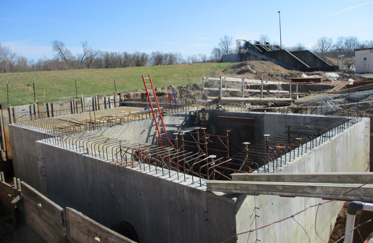
Stormwater Pump Station No. 1 - Photo 1
