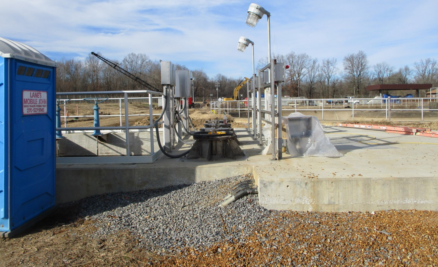
Nitrate Pump Station - Photo 1
