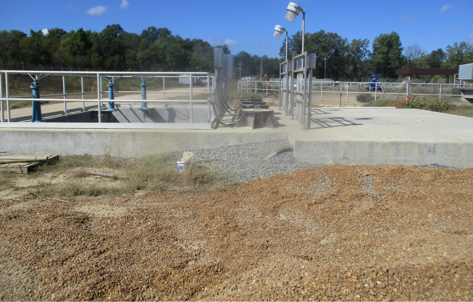
Nitrate Pump Station - Photo 3
