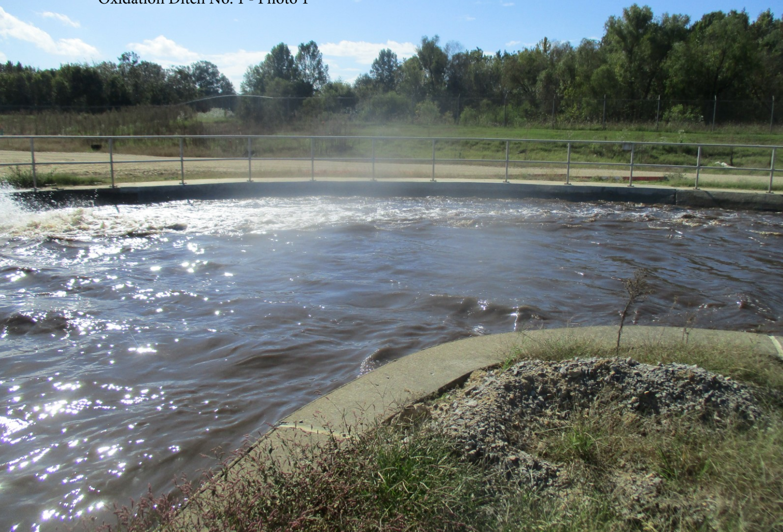
Oxidation Ditch No. 1 - Photo 1
