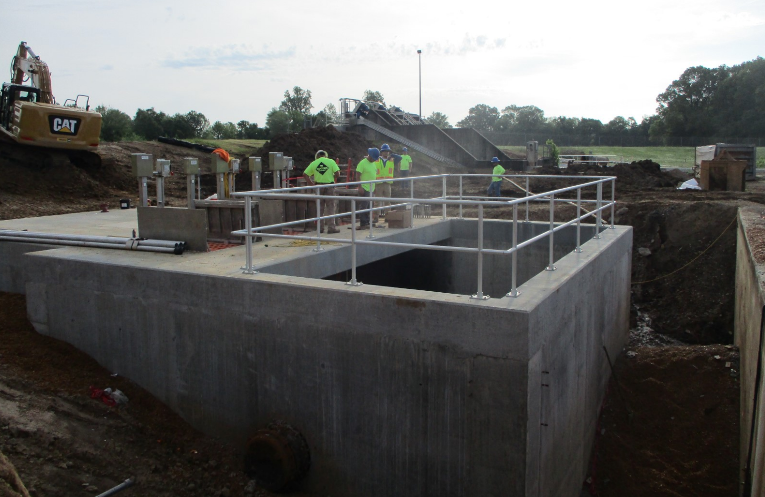
Stormwater Pump Station - Photo 1
