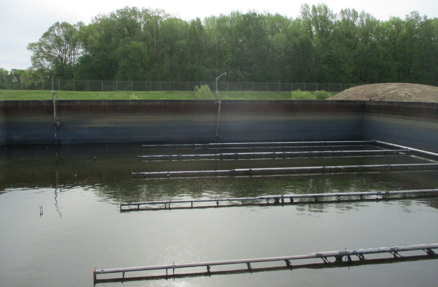
Interchange Tank - Photo 1
