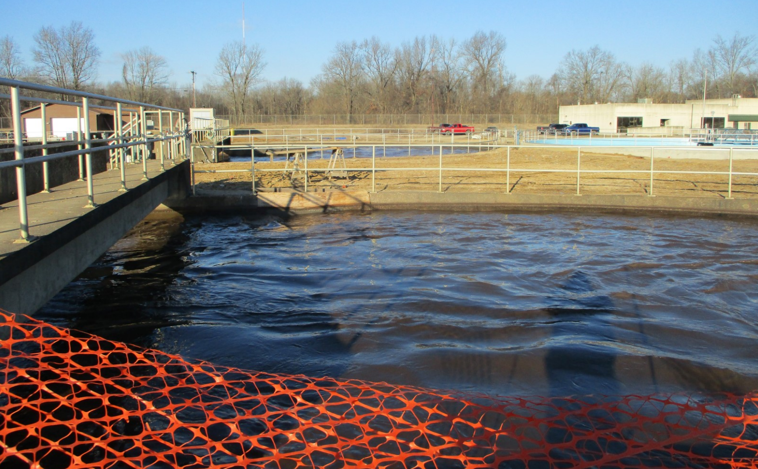
Oxidation Ditch No. 2 - Photo 3
