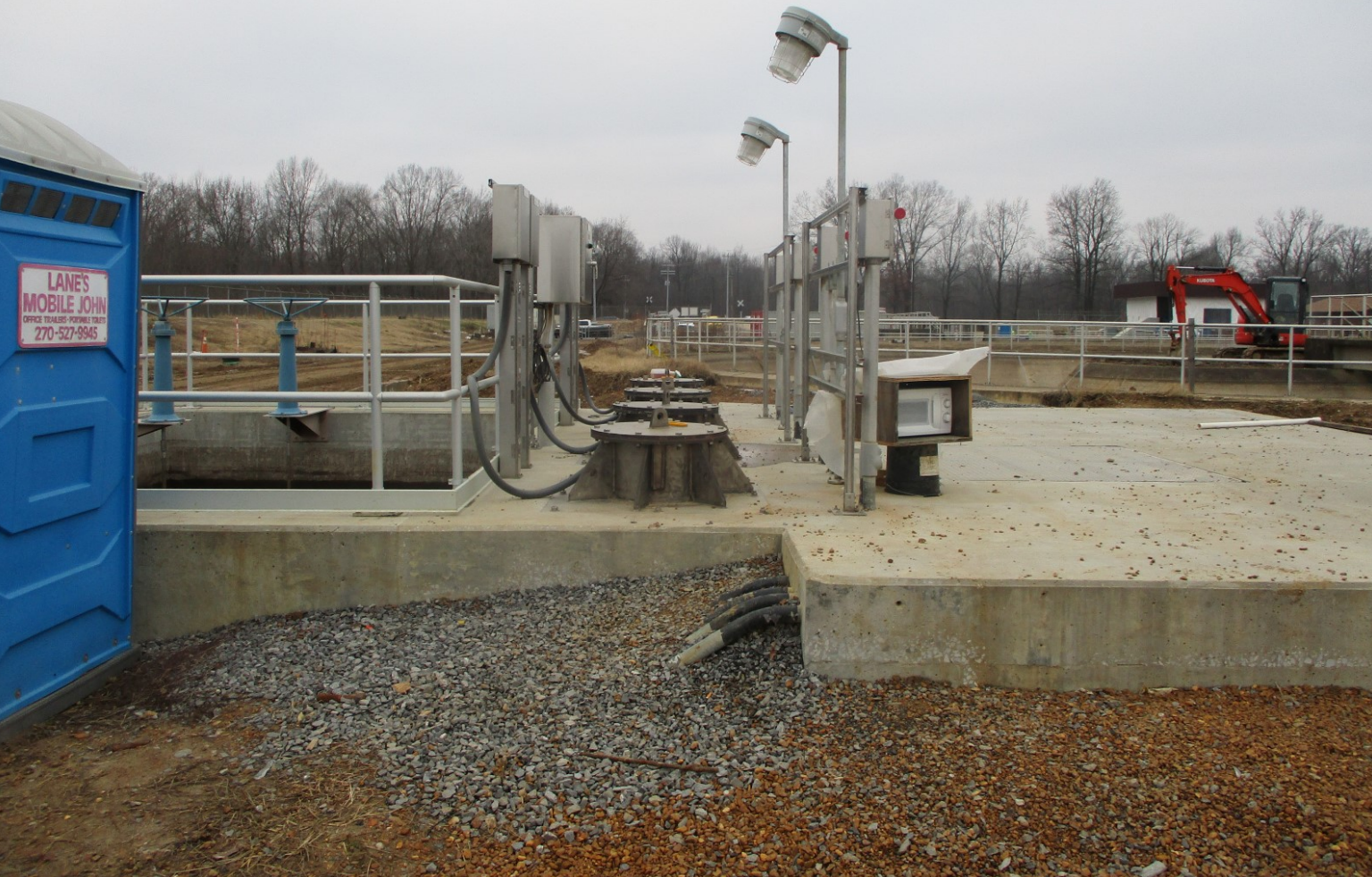
Nitrate Pump Station - Photo 1
